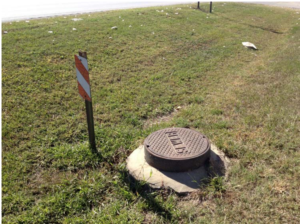
Figure 17: Sewer line running across the street along Hwy 82 on the front of the property.
